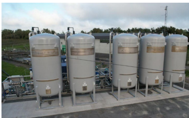
Horedown Water Treatment Works - Temporary Granular Activated Carbon Plant
