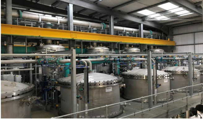
Figure 15: Mayflower Water Treatment Works (Photo Courtesy of PWNT)
